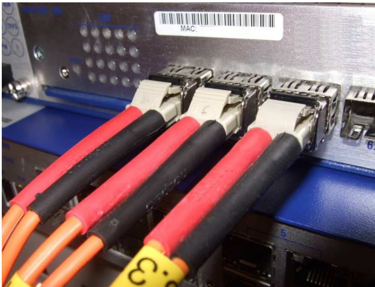
Figure 17 – Switch with optical fibres (LC connectors)
