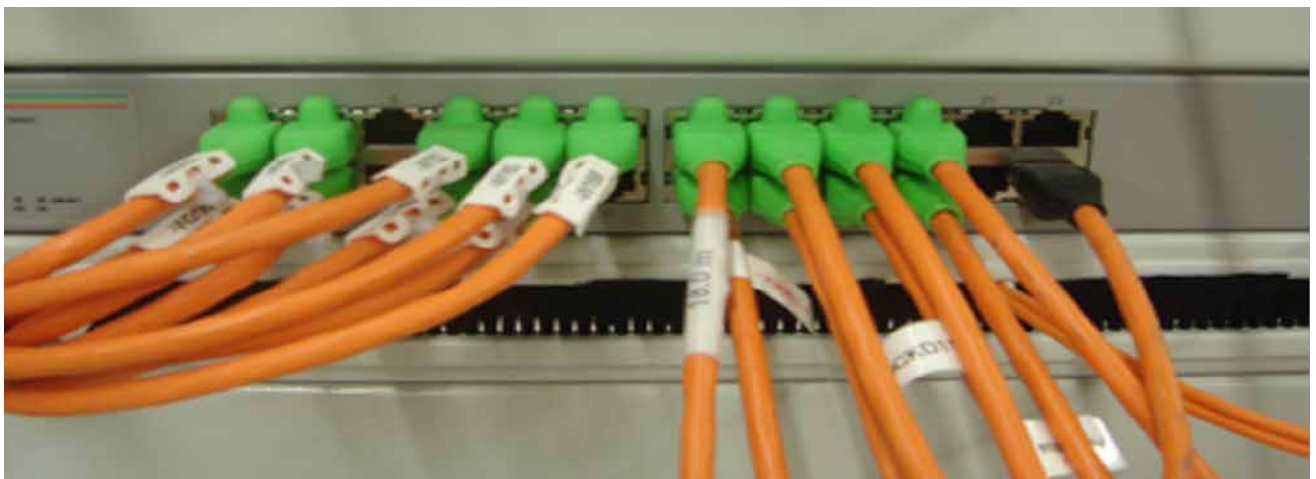
Figure 14 – Switch with copper (RJ45) ports)
